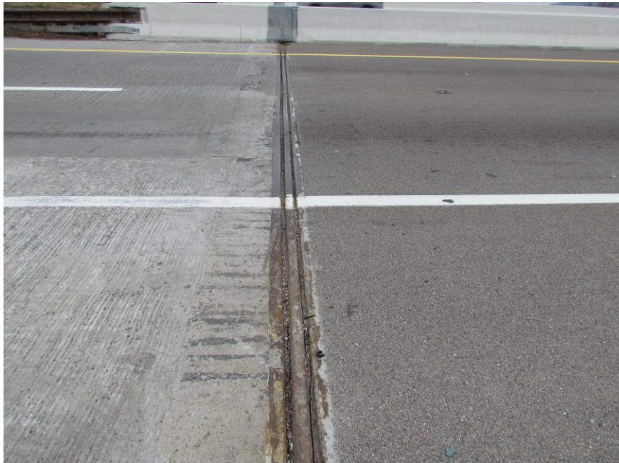
APPR. "B" JOINT W/ DEBRIS BLD-UP
