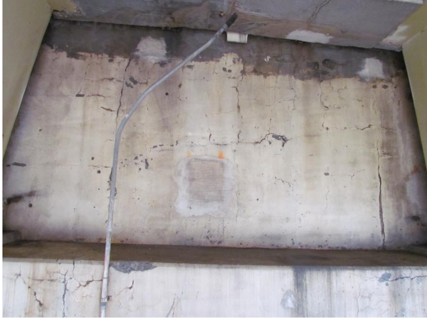
BACKWALL ABUTMENT #1 W/ MAP CRACKING
