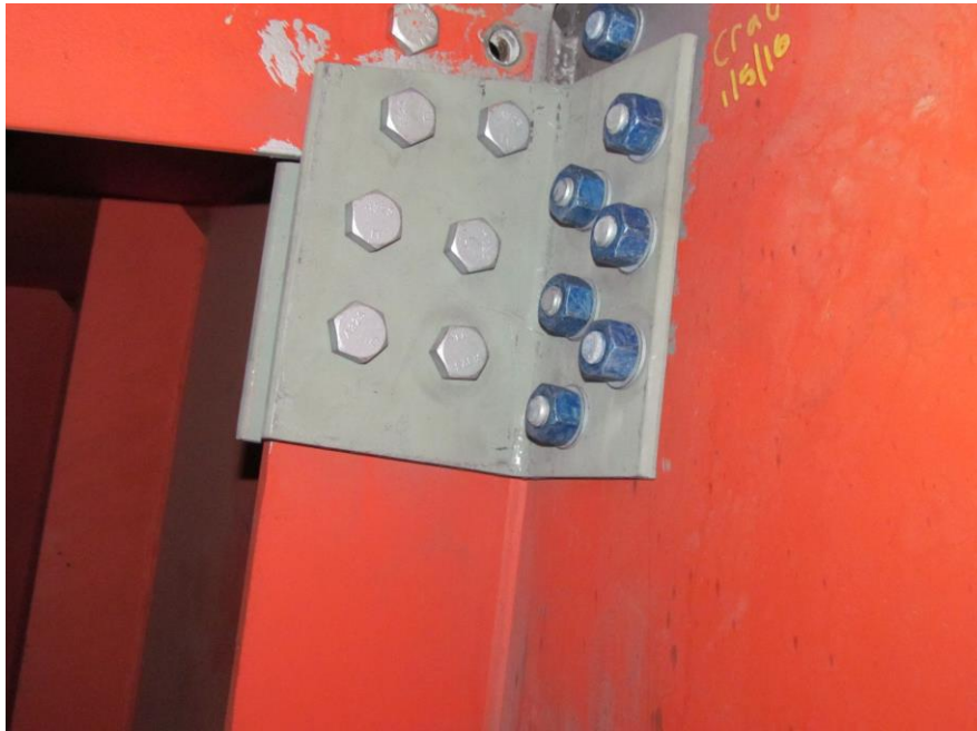
TUB "B" SP. #4 DIAPH. # 6 W/ 1 MISSING BOLT
