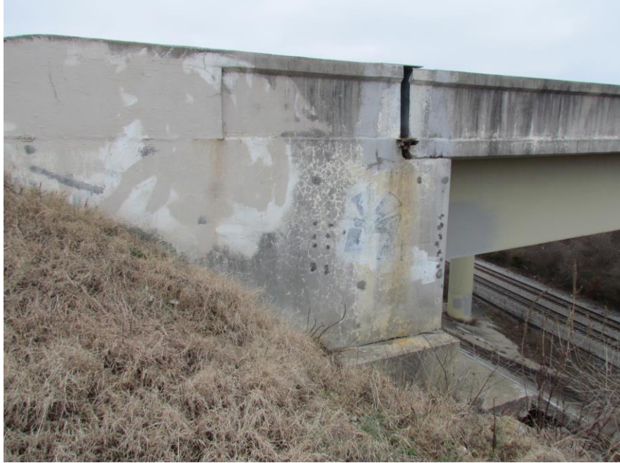
ABUTMENT #2 LT. WING W/ MAP CRACKING
