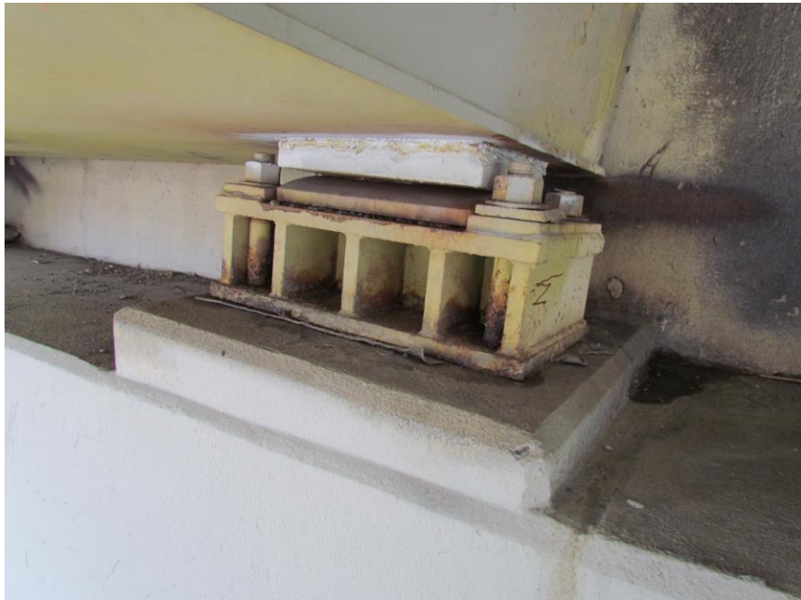
BEARING DEVICE "B" ABUTMENT #2 W/ CORROSION
