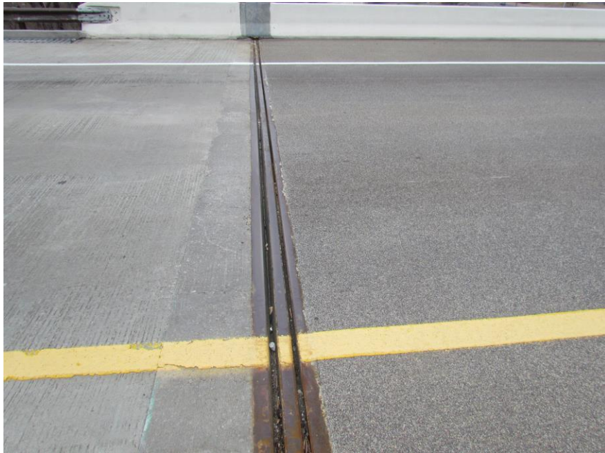
APPR. "A" JOINT W/ MEMBRANE FAILURE
