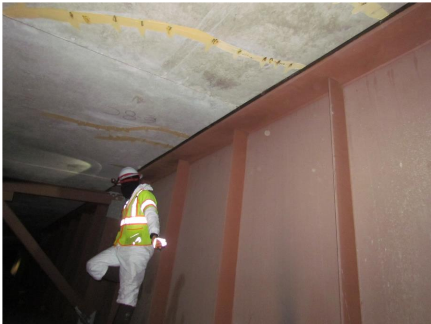
TUB "B" DECK PANEL SP. #6 W/ REPAIRS
