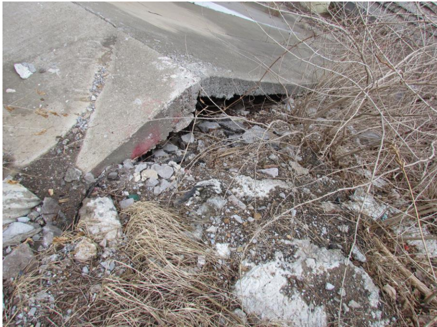
EMBANKMENT ABUTMENT #2 W/ EROSION
