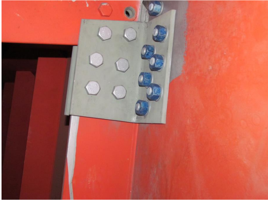
TUB "B" SP. #4 DIAPH. #5 W/ 1 MISSING BOLT
