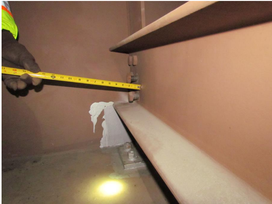
TUB "B" SP. #5 STIFFNER W/ 2 LOOSE BOLTS
