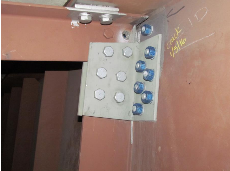
TUB "B" SP. #5 DIAPH. #5 W/ 1 MISSING BOLT
