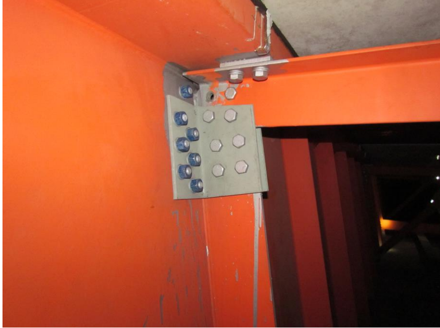
TUB "B" SP. #3 DIAPH. #6 W/ 1 MISSING BOLT
