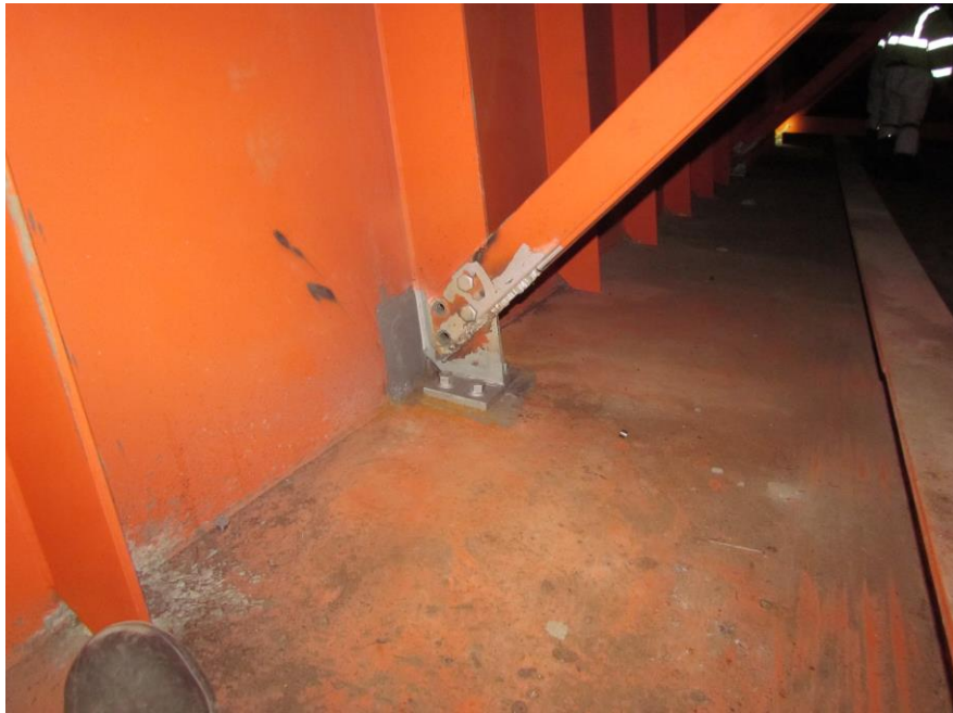
TUB "B" SP. #2 DIAPH. #6 W/ 2 MISSING BOLTS
