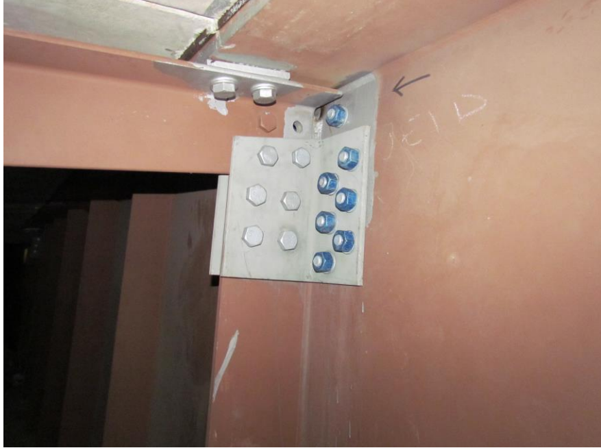
TUB "B" SP. #5 DIAPHRAGM W/ 1 MISSING BOLT
