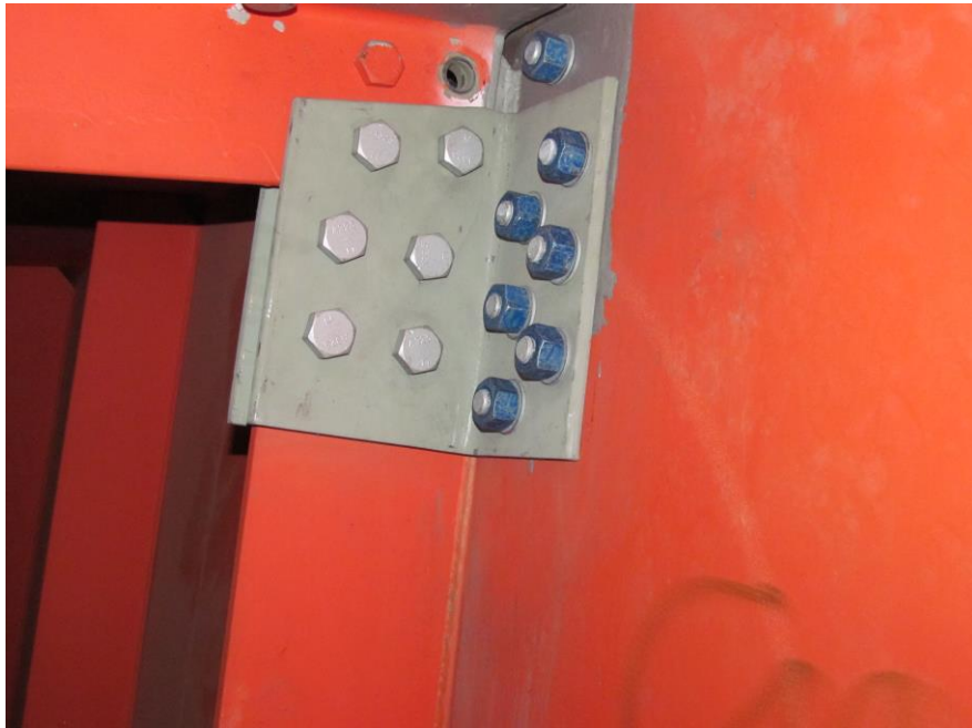
TUB "B" SP. #4 DIAPH. #3 W/ 1 MISSING BOLT
