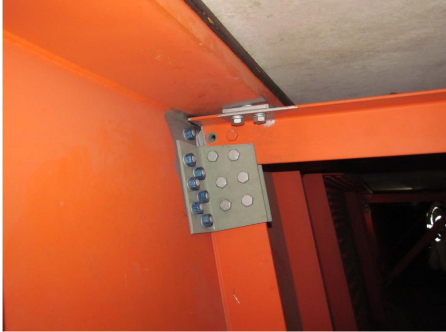
TUB "B" SP. #3 DIAPH. #4 W/ 1 MISSING BOLT
