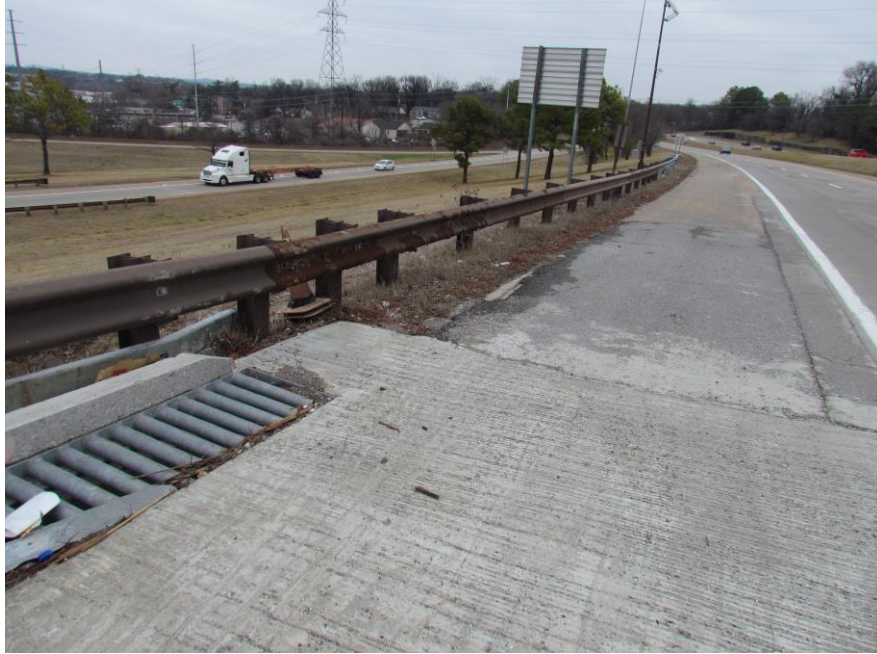
GUARDRAIL "B" LT. SIDE W/ CORROSION
